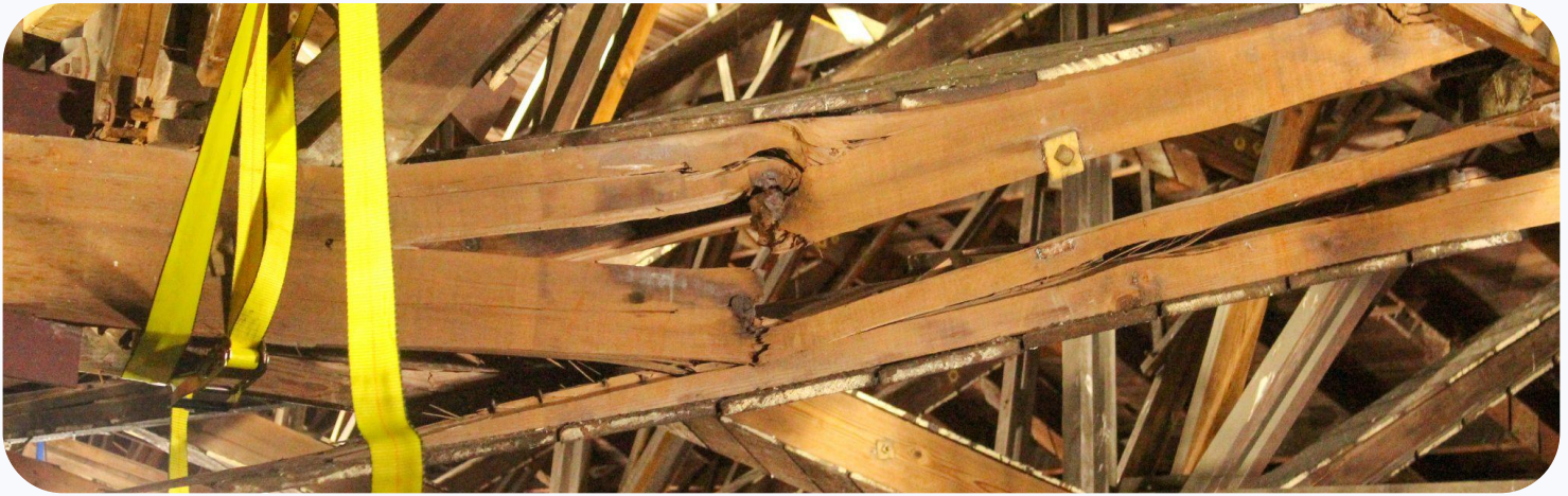
Damaged wooden beams within a complex truss structure, secured with yellow straps.
